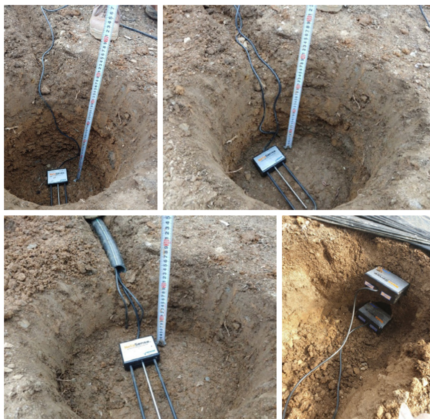
Figure 5. Sequential installation of three Netasense soil moisture sensors in the excavated pit on the top of each other and two sensors in the side wall of the excavation (bottom right)
